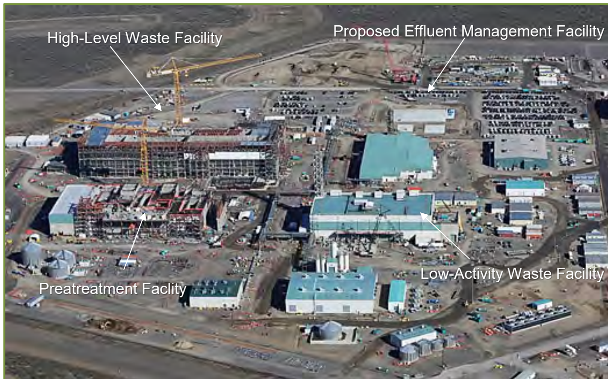
The Waste Treatment Plant, commonly called the vit plant, in 2016 (photo courtesy of Bechtel).
