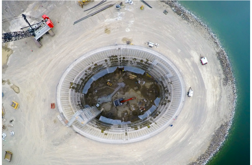
Construction of a vault to house a juvenile fish passage helix structure at Cle Elum Dam.
