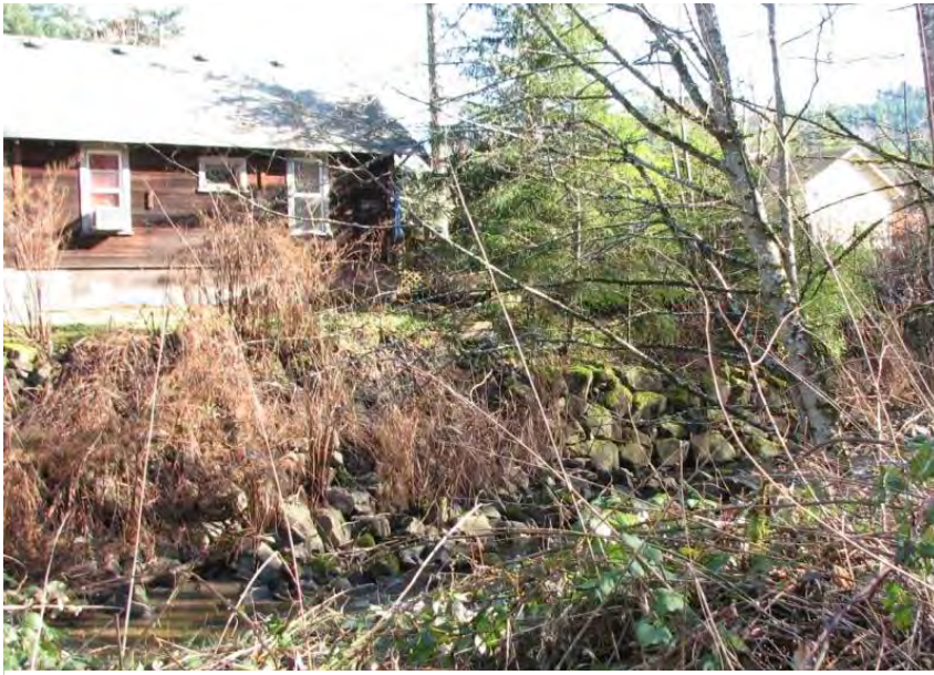
Photo 5: Reach 1c: Photo on left is incised channel in Reach 1c. Riprap is evident on stream right. Some is failing.
