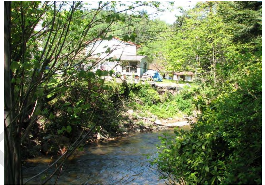
Photo 6: Reach 2a: View downstream at incised channel. Bank erosion is occurring on stream left.
